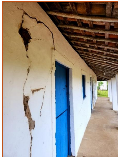
Image 5: Side facade of the MLLC, highlighting the crack in the wall. Photo by the author, 2025.
